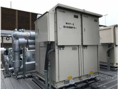
Heat pump that use river water
