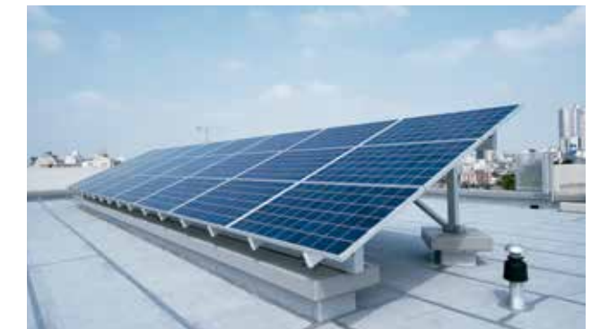
Photovoltaic generation system panels (Sunny Life Tokyo Shinjuku)
