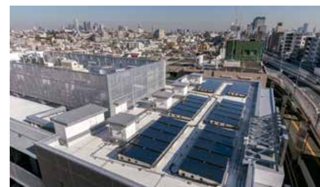
Solar heat collection panels (Hulic Setagaya)
