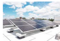
Photovoltaic panels installed on the rooftop of Hulic Fukasawa
