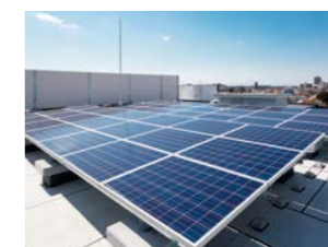
Photovoltaic panels (Hospitalment Itabashi Tokiwadai)
