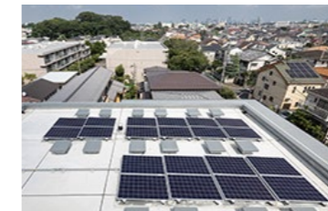
Photovoltaic panels installed on the roof top of Trust Garden Ogikubo
