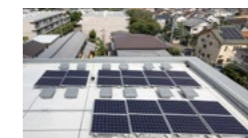
Photovoltaic panels on the roof
