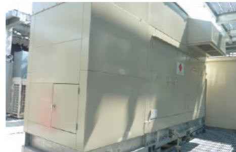
Emergency back-up generator
