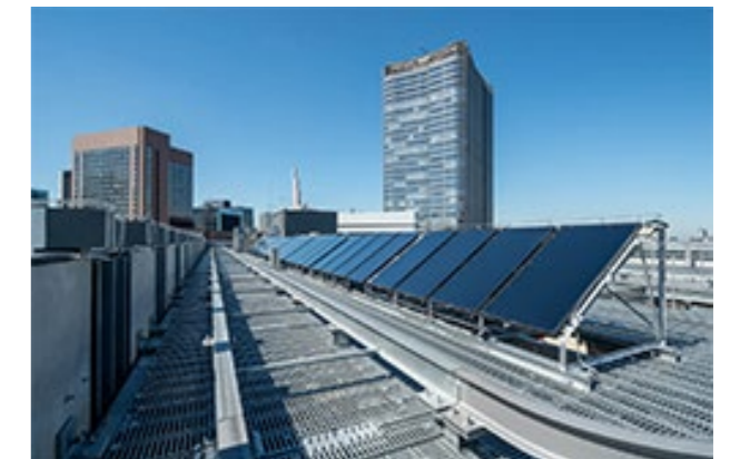
Solar heat collection panels (HULIC SQUARE TOKYO)
