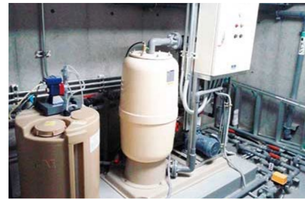
Rain water reutilization equipment at HULIC Setagaya
