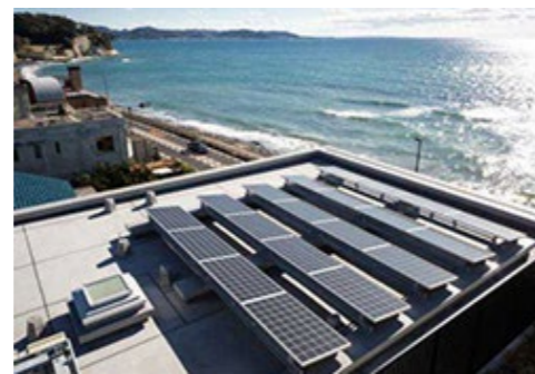
Photovoltaic panels on the rooftop (Granda Inamuragasaki Kamakura Aoitei)
